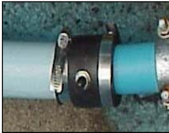
Test boot located in a sump
