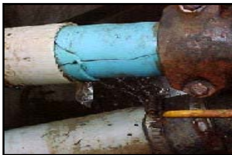
Flexible piping is cracked
