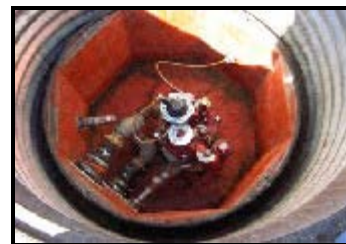
Contained turbine sump
