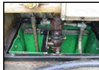
Contained dispenser sump
