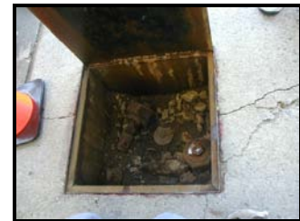
Square steel sump lid pulled up to show the inside of an uncontained turbine sump
