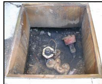
Uncontained turbine sump
