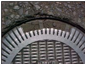
Cracked spill bucket lid
